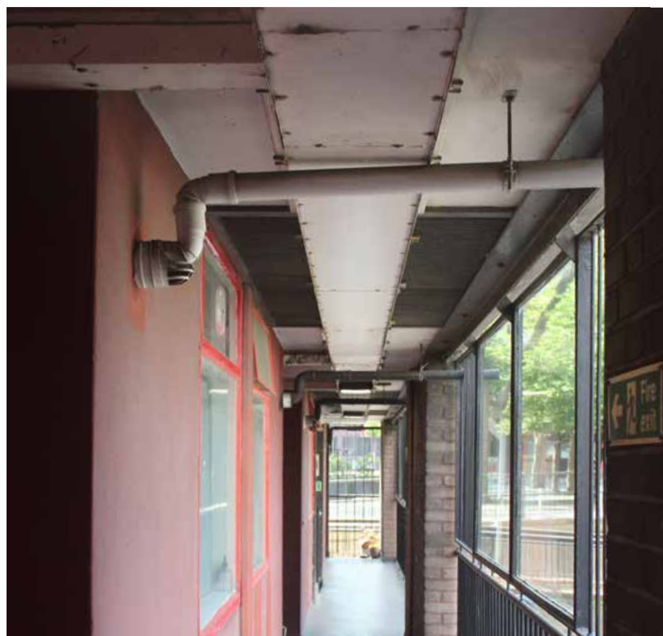
Existing horizontal and vertical services distribution in communal areas
