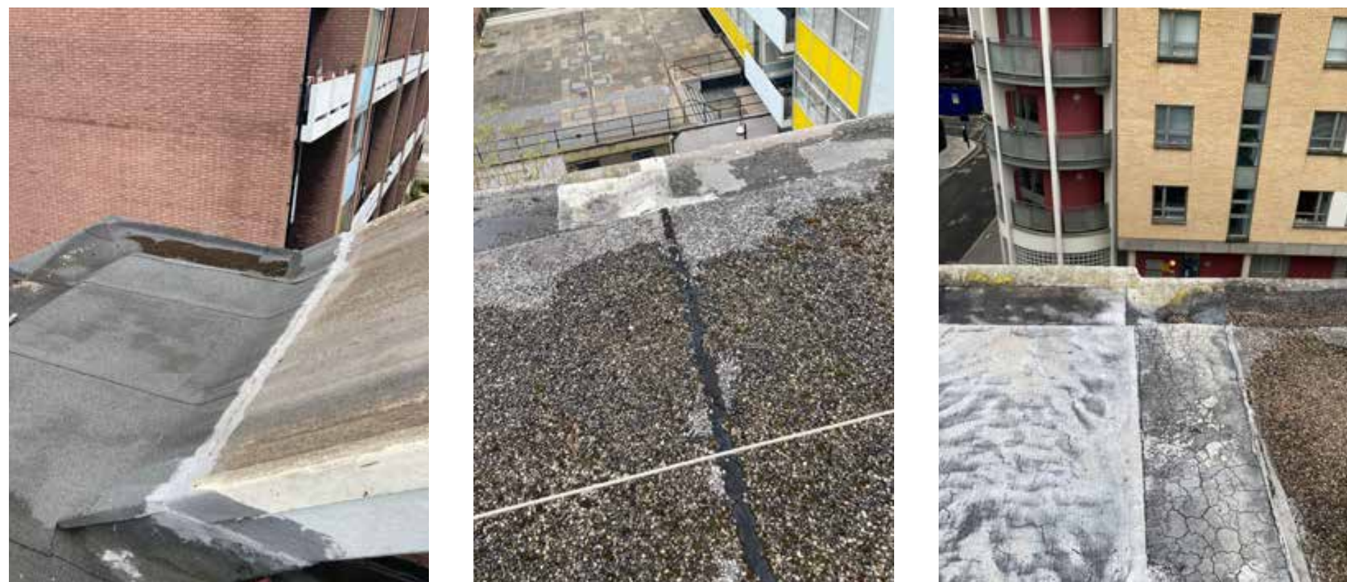
Detailed photos showing conditions of the Cuthbert Harrowing House roof showing pooling water, patch repairs, joints in finishes and aging coverings.
