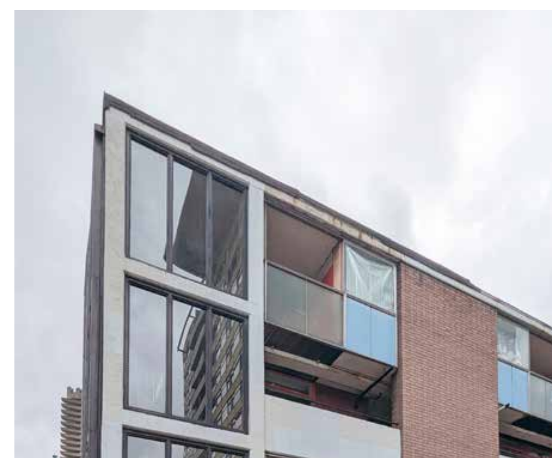
The crisp edge of the roof has been lost over time following addition of new coverings.
