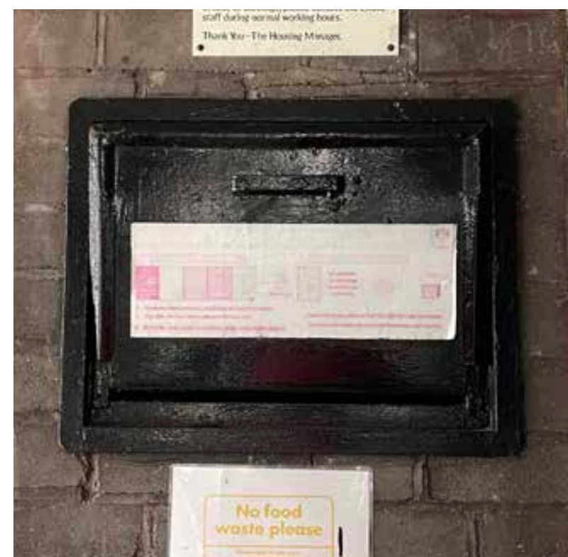
Existing refuse chute hopper
