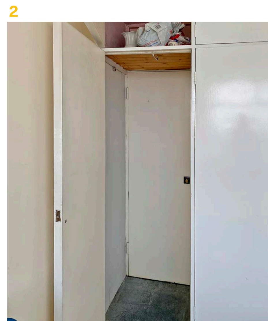
The cupboard escape routes to middle flats are often obstructed - residents may not be aware of their purpose.
