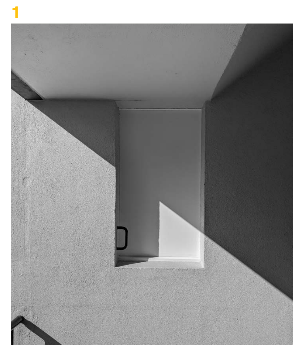
The escape hatches are 1.5m above the stair and are not very practical.
