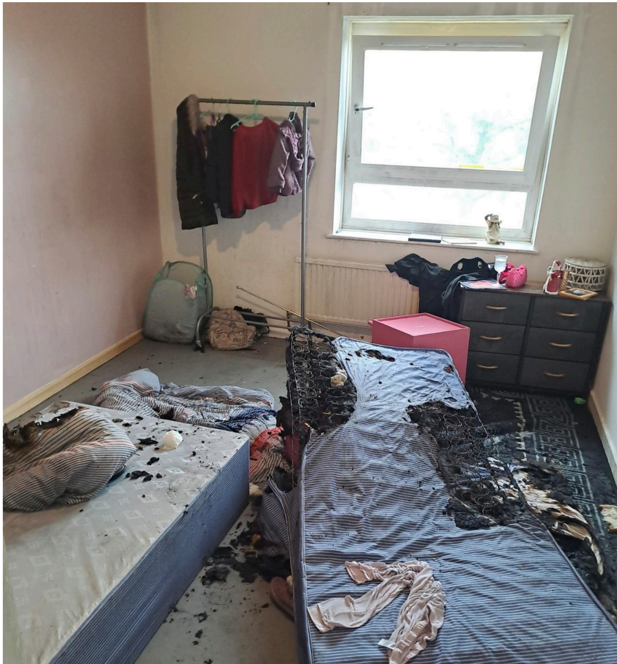
A fire which occurred in a tall residential building was contained and extinguished by the activation of the building's sprinkler system.
