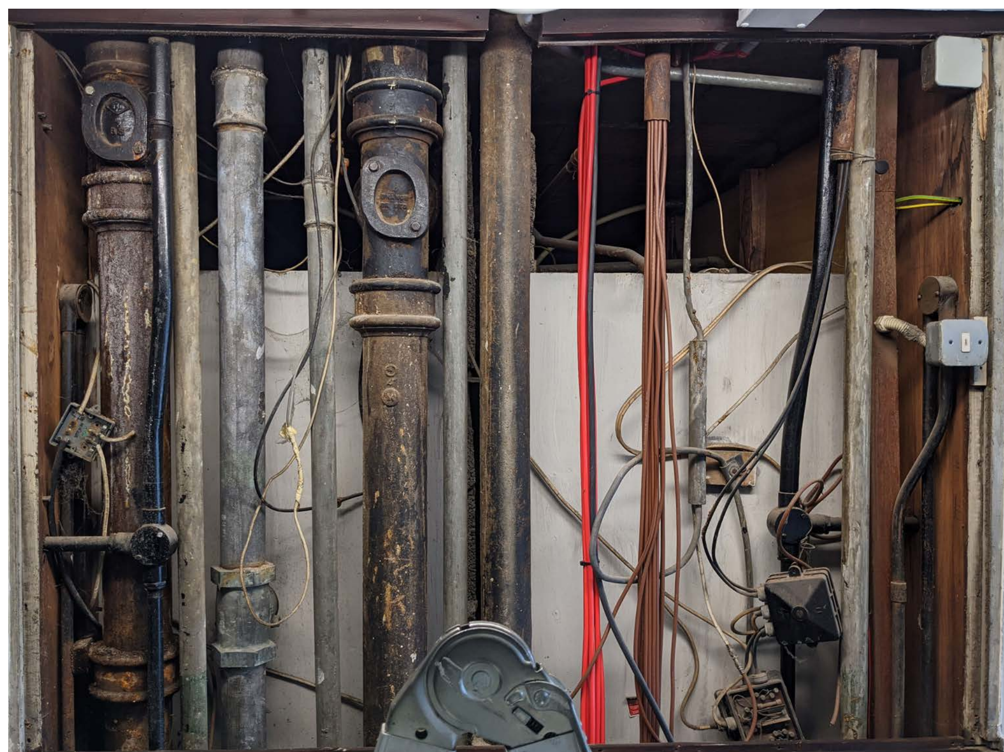
Risers contain: gas, water, electricity, telecommunications, rainwater and foul drainage services.
