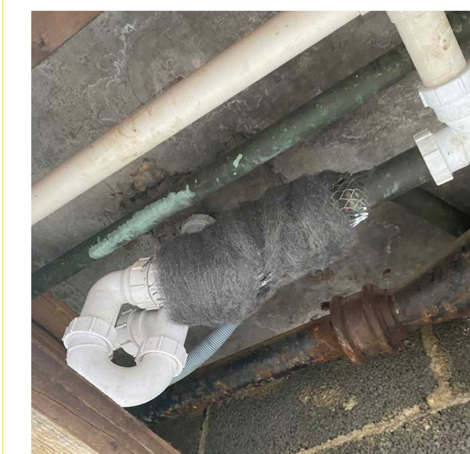
Plastic UPVC repair with wire wool wrapped around the pipework.
