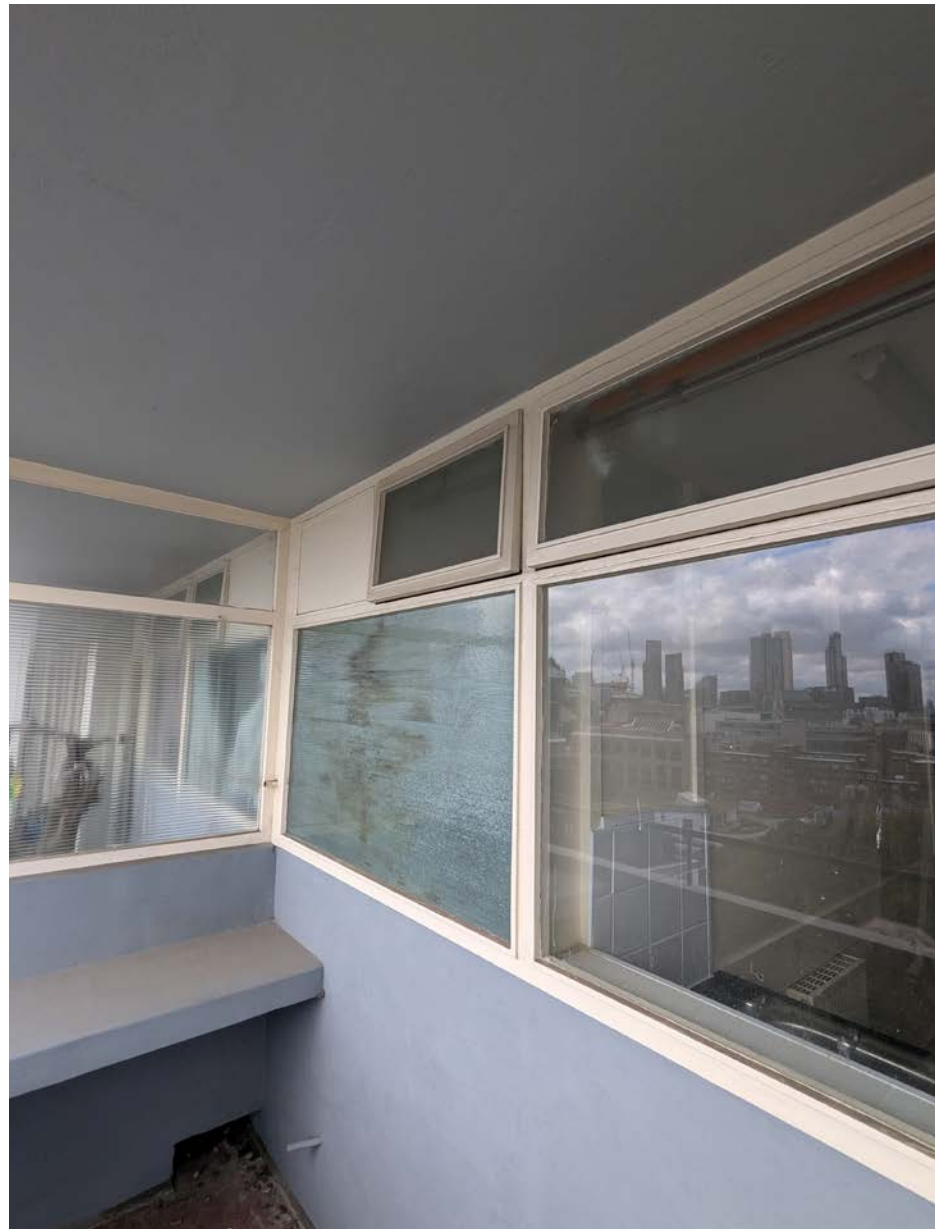
Timber-framed kitchen and bathroom windows. The top-hung opening windows sit proud of the frame when closed.
