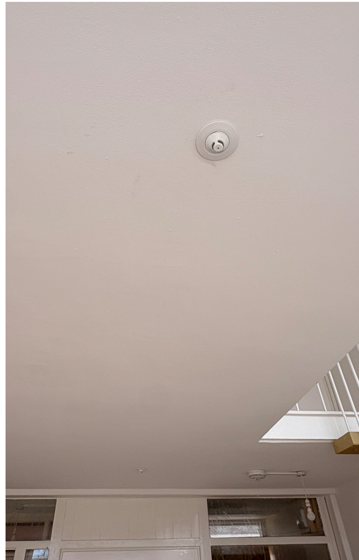
Trial mist suppression installation at 2 Bayer House. The recessed head has pipework concealed within the ceiling.
