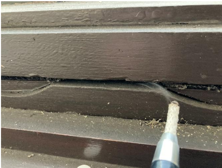
Photograph 16: Air Leakage - window frame (SAL14)
