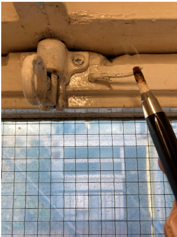
Photograph 6: Air Leakage - kitchen window (SAL4)
