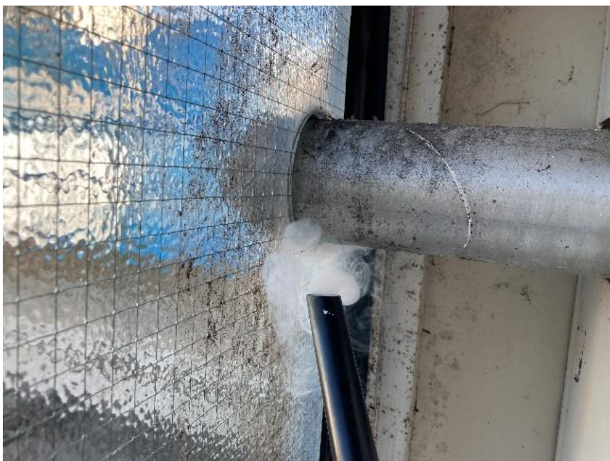
Photograph 8: Air Leakage – bathroom flue (SAL6)
