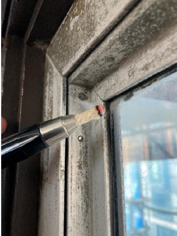
Photograph 11: Air Leakage - window frame (SAL9)
