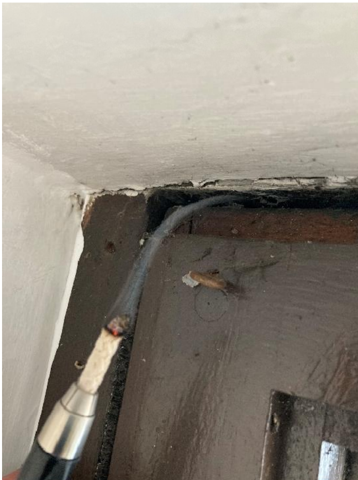
Photograph 14: Air Leakage - window frame (SAL12)
