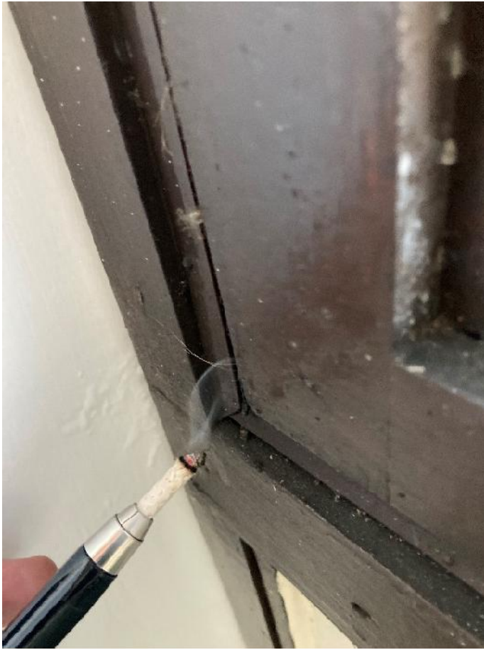
Photograph 15: Air Leakage - window frame (SAL13)
