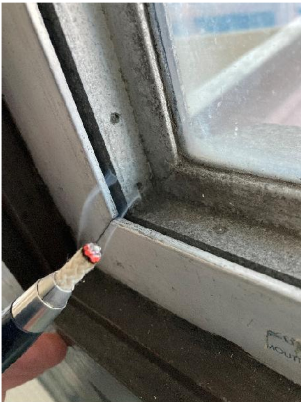
Photograph 12: Air Leakage - window frame (SAL10)
