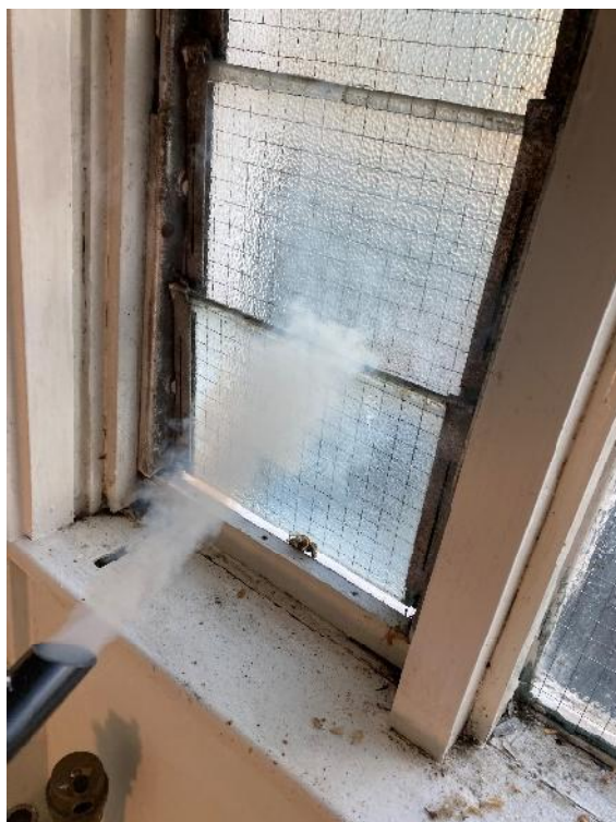
Photograph 7: Air Leakage – bathroom louvre (SAL5)
