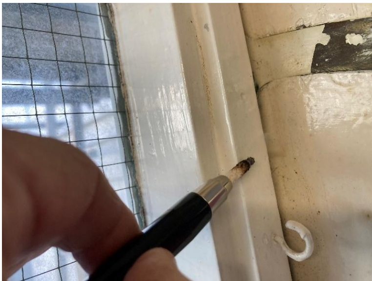
Photograph 4: Air Leakage - kitchen window (SAL2)
