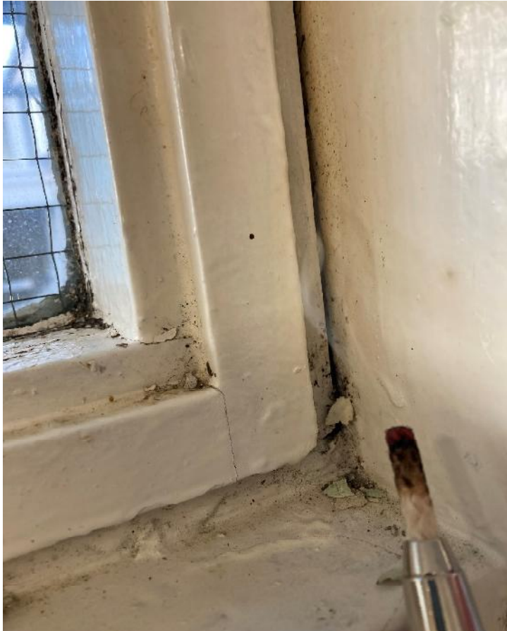
Photograph 3: Air Leakage - kitchen window (SAL1)
