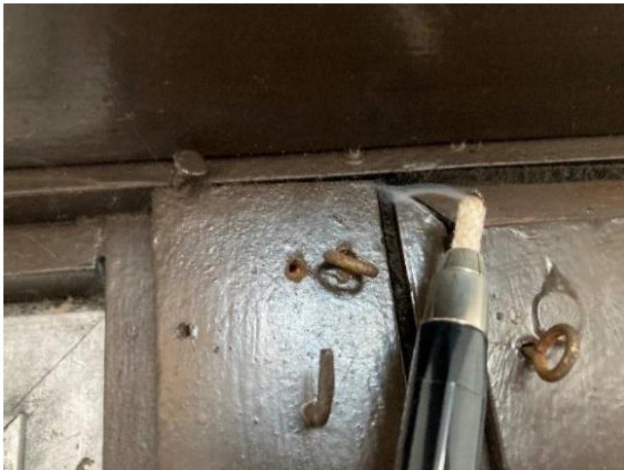
Photograph 10: Air Leakage – window frame (SAL8)
