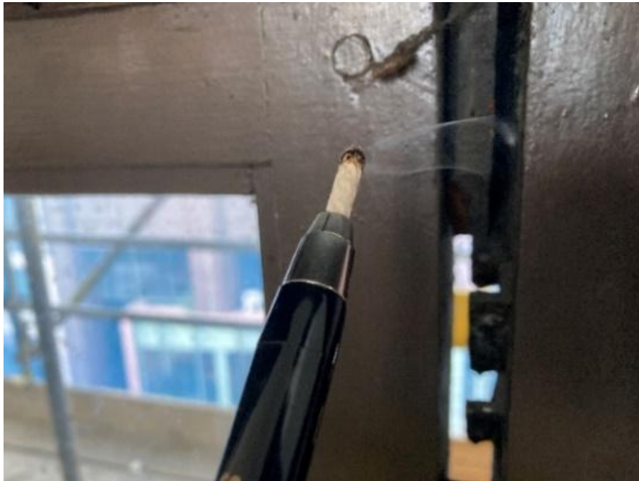
Photograph 9: Air Leakage – main window frame (SAL7)
