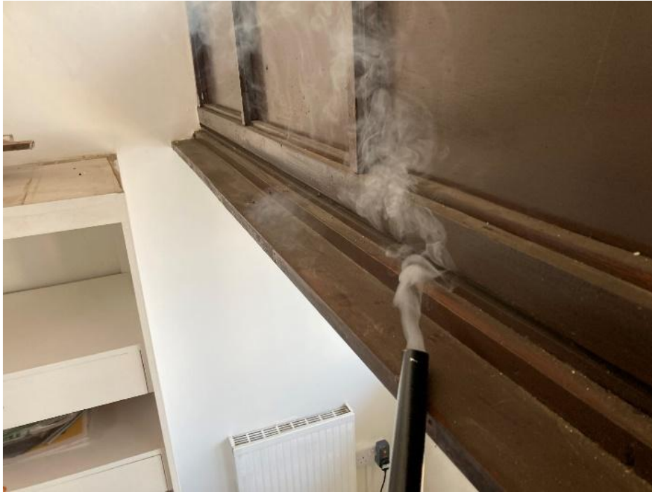
Photograph 13: Air Leakage - window frame (SAL11)
